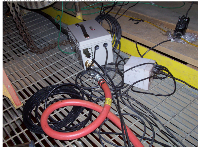
Figure 4 shows the air assist box with air lines and cables.
