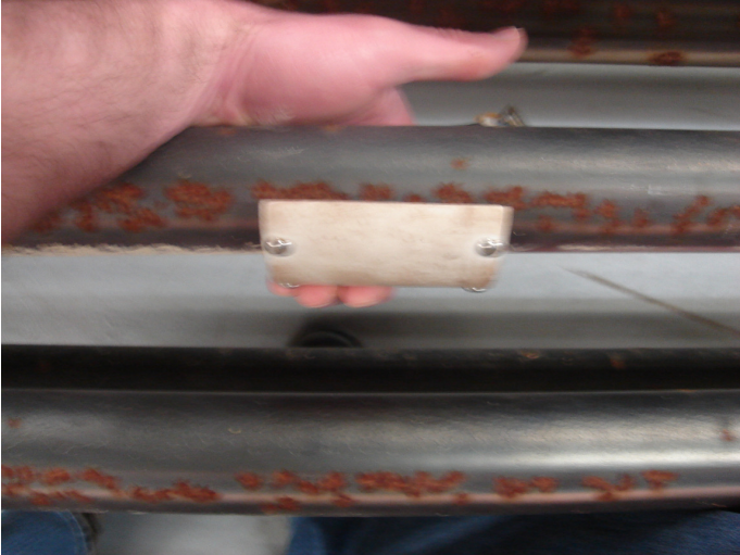
Figure 7 shows the Low Profile LFET scanner in a reheat bank.
